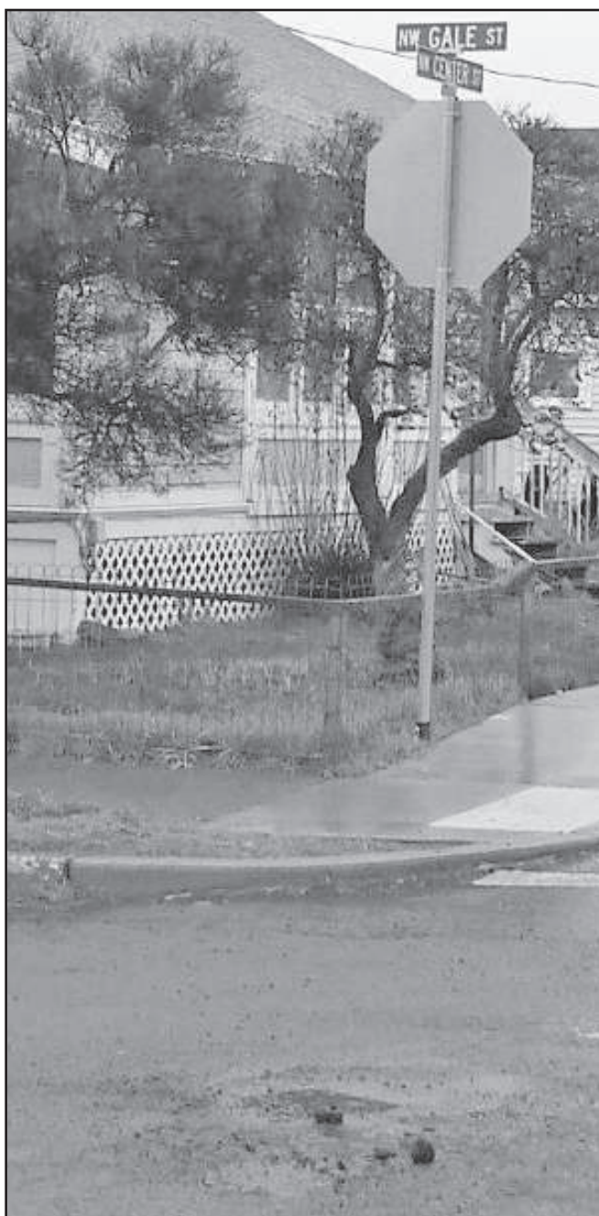
Gale Street is in need of repair to fix multiple potholes.
