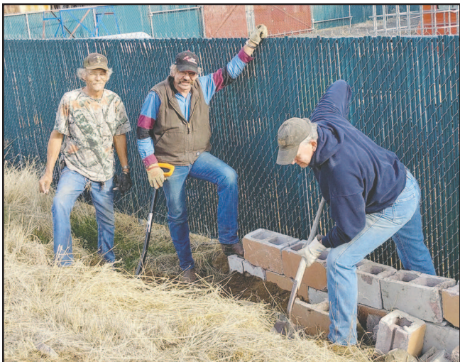
Lexington city maintenance manager Ed Dickenson and town council members' spouses Reid Miller and Wayne Gordon help build a retaining wall in the FEMA park on Main St. in Lexington. -Photo by Bobbi Gordon
