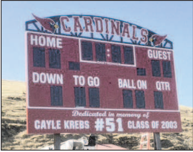
The Ione School District, with the donated help of manpower and equipment from Port of Morrow, Columbia Basin Electric and Loyal Burns installed a new scoreboard at the football field. The score board was purchased with donations in memory of Cayle Krebs. -Contributed photo
