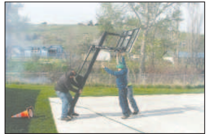
Heppner city workers replace the basketball hoops at Hager Park, which had to be taken down, rewelded and put back up after they were damaged in a recent rash of vandalism at city parks. -Photo by David Sykes
