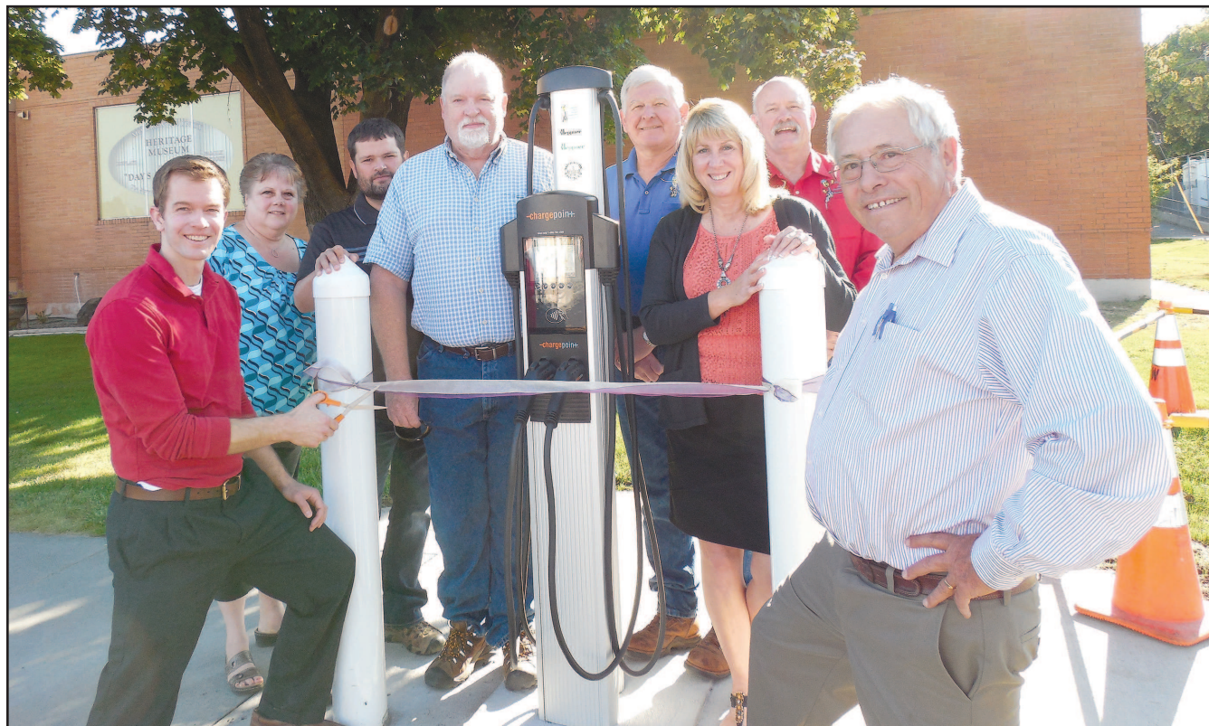
Columbia Basin Electric Cooperative finished installing a new electric vehicle charging station in Heppner recently. The station was the last of four installed in the co-op's service area, with others located in Ione, Condon and Fossil. Celebrating the car charging station opening with a ribbon cutting Monday were (L-R) Morrow County Administrator Jerry Sorte, Heppner Chamber of Commerce Executive Director Sheryll Bates, CBEC Assistant Manager of Operations Josh Coiner, Heppner Mayor Skip Matthews, CBEC Board Member Gerry Arnsen, CBEC Staff Accountant Debbie Lankford, CBEC General Manager Tommy Wolff, and Morrow County Judge Terry Tallman. -Photo Andrea Di Salvo
