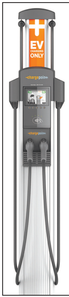
Electric car charging stations like this are set to be installed not only in Heppner and Ione, but also in Condon and Fossil. -Contributed photo
