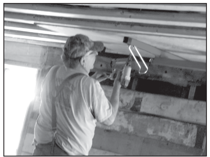
Mel McDaniel gets going on the ceiling in Hardman Community Center. -Contributed photo
