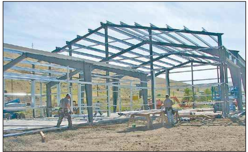
With the foundation laid, the new fire hall in Heppner is going up by leaps and bounds. The hall is estimated to be complete in late August. -Photo by David Sykes
