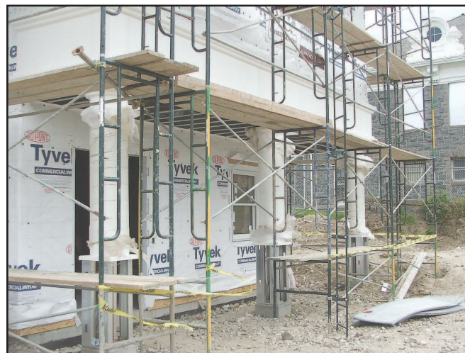
Columns along the side are just one of the ways the new building is "blended" into the older existing courthouse. —Photo by David Sykes
