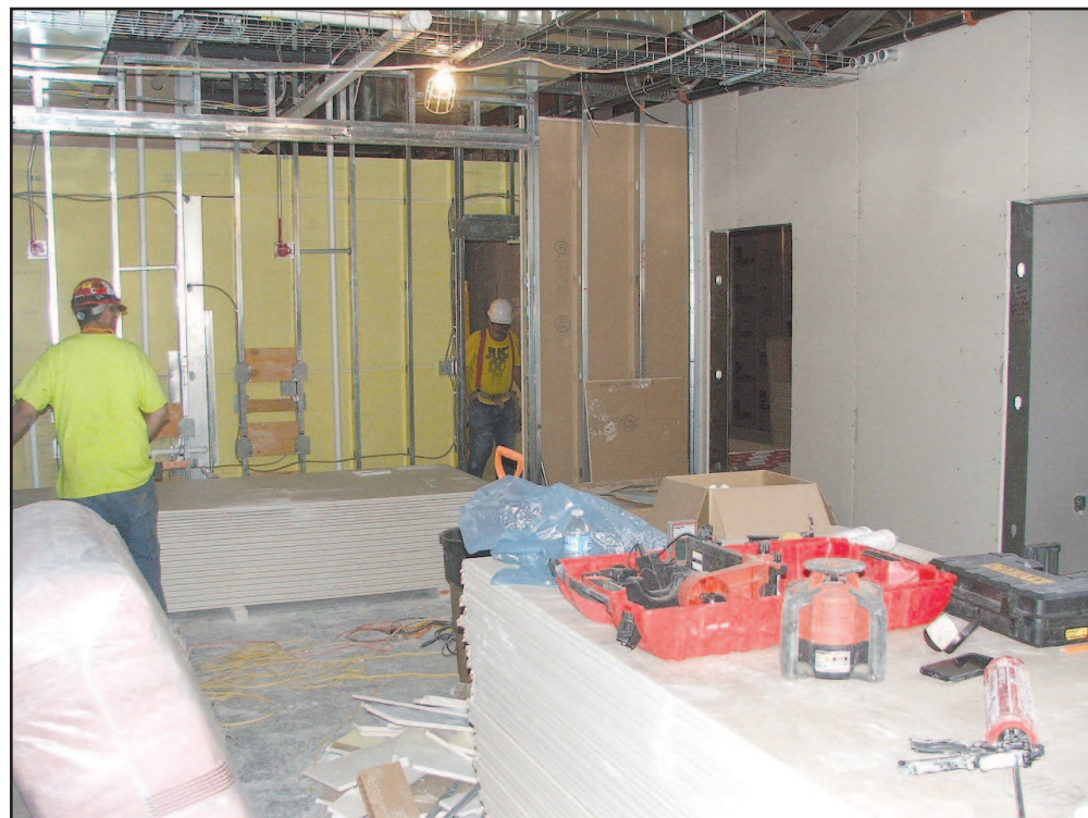
Workmen have been busy inside the new Bartholomew Building adding sheetrock, electrical, plumbing and other infrastructure in preparation for the scheduled October completion date. Studs are all metal in this facility, explains construction superintendent Pat Post. —Photo by David Sykes
