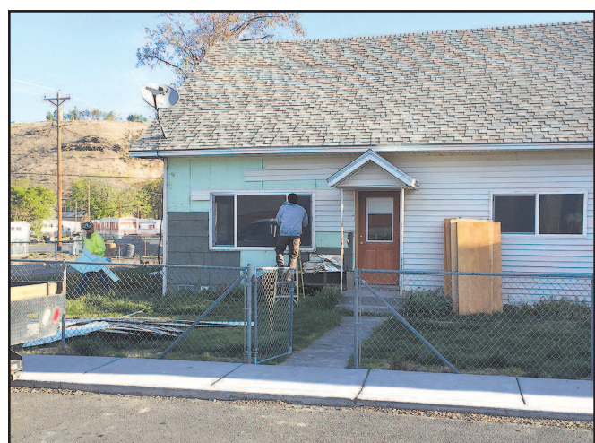
Knerr Construction started the remodel of the Ione Community Clinic at 325 E. 3 rd street this week. This will be a school-based health clinic open to the whole community, staffed 20 hours a week through a partnership of Morrow County Health District, Morrow County Public Health, Community Counseling Solutions and Advantage Dental. Grants for the building and remodel were received from the Ione Education Foundation and ICABO with further grants pending from Oregon Community Foundation, Ford Family Foundation, Columbia River Enterprise Zone, and Wildhorse. Ione Community Clinic is set to open in August. -Contributed photo
