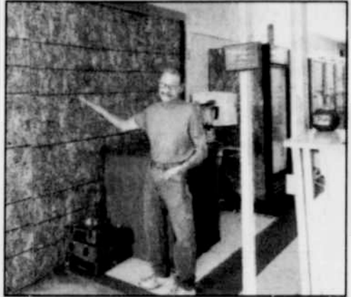
Ron Howe of Howe's About Pizza shows the plywood-covered hole where a car drove through the wall of his restaurant. -Photo by Andrea Di Salvo
