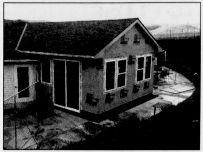
Residents and staff at Willow Creek Terrace hope the completion of this new addition will give them something to be thankful for this Thanksgiving. -Contributed photo
