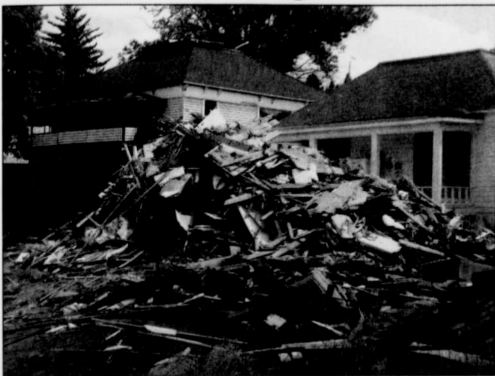
A house located next to the Morrow County Courthouse is now just a pile of rubble. As of Tuesday morning, workmen had finished tearing down one of the three houses that will be demolished in the coming days to make way for construction of the new county administration building. The new 10,000-square-foot facility will be built to house the Morrow County Health Department and some other county agencies. The new building is being built right next to the existing courthouse, which will still have many county services located there. -Photo by David Sykes
