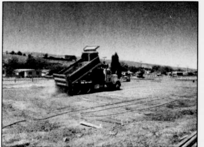
A new basketball court under construction on Riverside St. in Heppner (above) has received a boost in funding in the form of a $10,000 grant from the Wildhorse Foundation. Willow Creek Park District is managing this project; the low bid for construction of the project came from Dice Construction. Dice broke ground the week of May 26, and they expect to pour concrete by the third week in June. The court will be a concrete slab, with high-end 72" hoops, lighting, striping, fencing and landscaping. The City of Heppner will be assisting with the administration of this project but will not be funding it. This project has been made possible through volunteer efforts and community support. -Contributed photo
