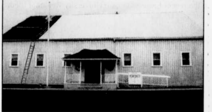
The Ione American Legion Hall received a new roof recently thanks to community support. -Contributed photo
