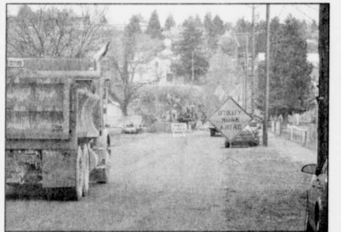
A portion of Chase St. will be closed for a couple of weeks for sewer repairs, the City of Heppner announced this week. -Photo by Andrea Di Salvo
