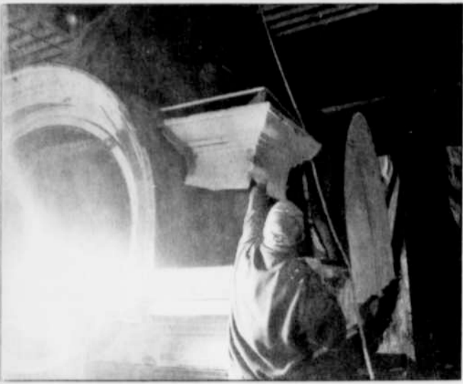
Rod Wilson displays how a piece of preserved tin will be refitted onto the clock tower once repairs are made. -Photos by Mallorie Jones
