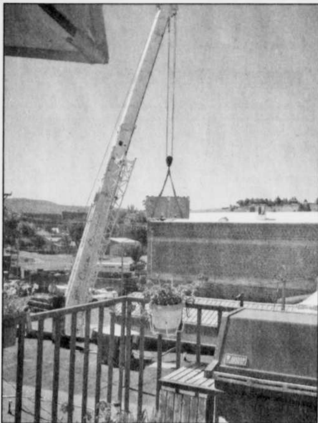
St. Patrick's Senior Center in Heppner received a long-anticipated new HVAC (heating, ventilation, and air conditioning) unit last Friday. A crane lifted off the old unit, which had been in disrepair for many years, and placed the new one. The total cost of the project is $22,847.80; a portion of the funds was donated from the City of Heppner sale of a HUD house and from proceeds of the Friends Helping Friends Remembrance Walk. —Photo by Megan Fitter
