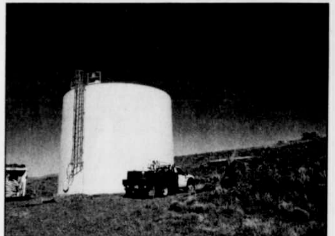
Heppner's water tank may need some major rehabilitation.
