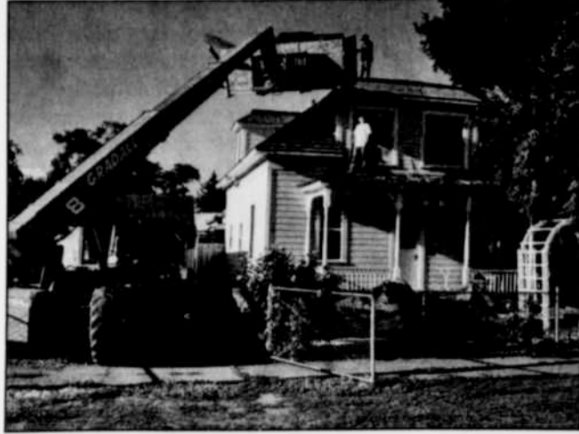
A new roof takes shape on the Shannons' home on the corner of Jones and Water in Heppner. The Shannons were able to replace their roof, among other things, with the loan money they received from the block grant. —Contributed photo
