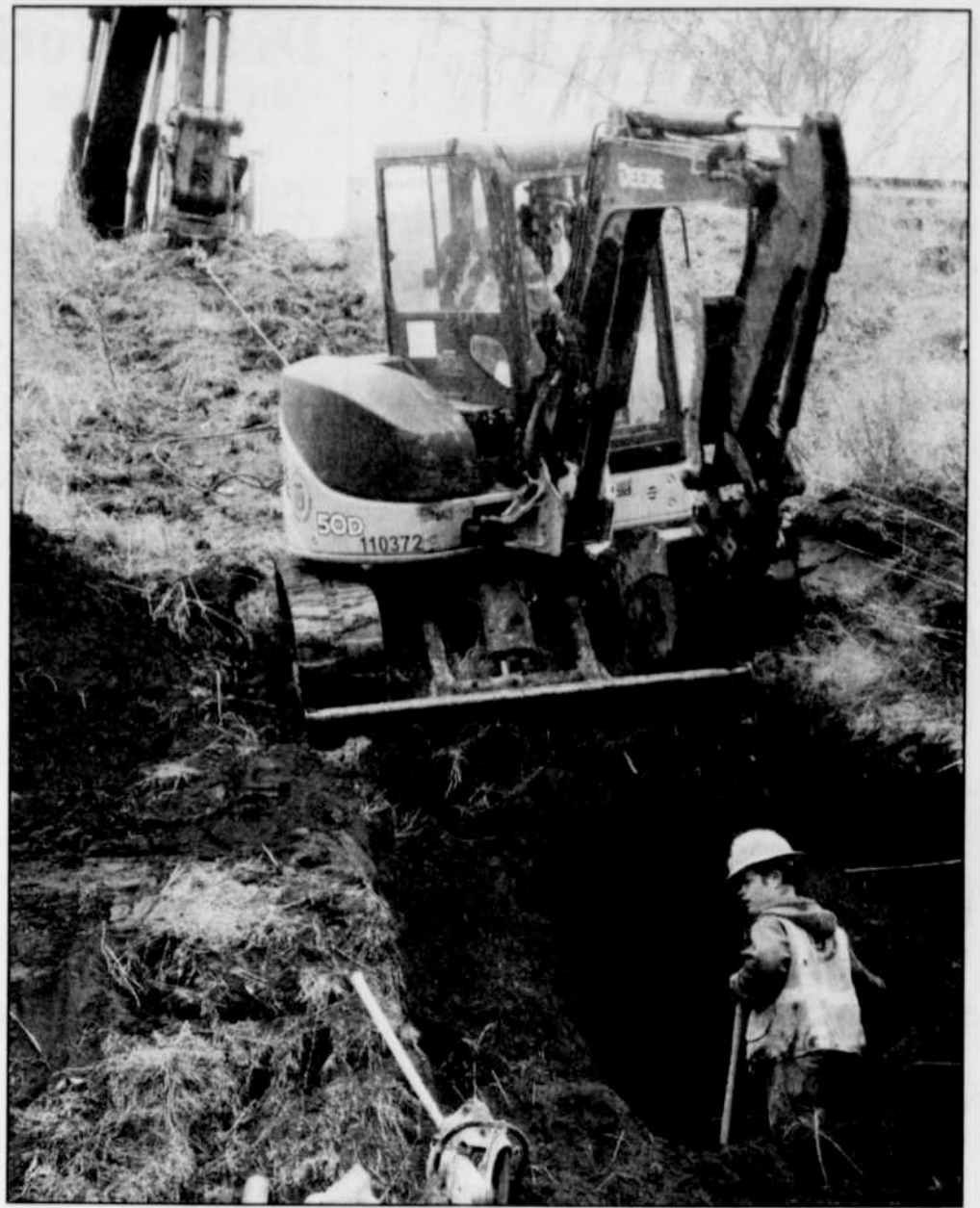
Work began Monday on the Barrett Blvd project in Heppner. Here, workers are beginning the excavation necessary to put in a drain pipe.
