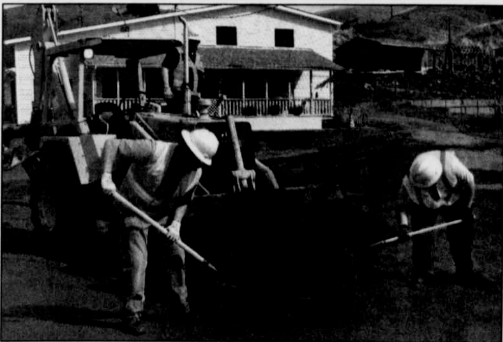
Heppner Public Works Director Brian Harmon works a front loader across from Green Feed as city crew members Michael Angell (left) and Robert Whalen clean up mud and other debris that washed down Linden Way in Heppner Monday night. —Photo by April Sykes
