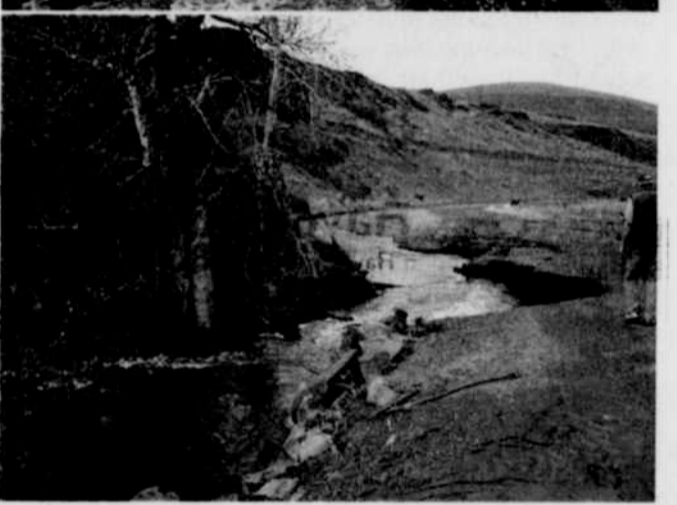
Recent rains have caused damage to some of the county roads. Such as this on Road Canyon.
