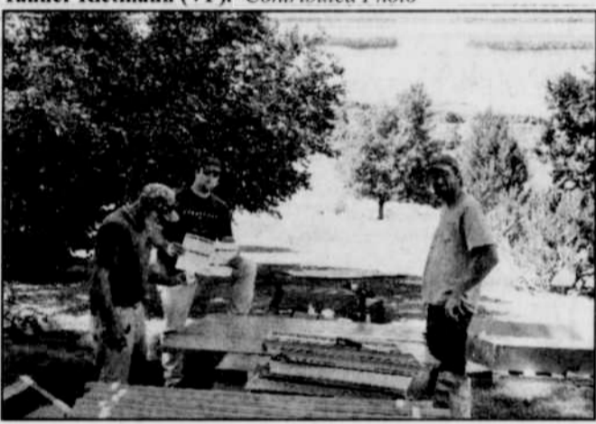
Volunteers Wayne Hams and Deacon Heideman assist city maintenance manager, Curtis Thompson, erect the gazebo in the Ione Community Park before the 4 th of July Celebrations. -Contributed Photo
