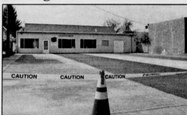
The Neighborhood Center of South Morrow County recently completed the replacement of their parking lot. Partial grant funds to complete this project were obtained from Wildhorse Foundation, Pendleton and Morrow County Discretionary Funds. J & G Concrete of Heppner completed this project with expertise and professionalism. On April 5 the parking lot will re-open to vehicles. Until then, visitors are asked to walk in. -Photo by Andrew Sykes
