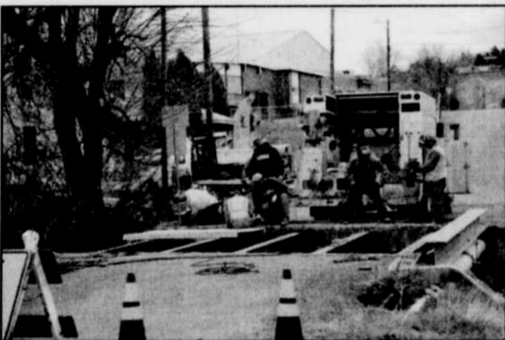
The Morrow County Road Crew reconstructed the Elder Street Bridge in two days. The project was a joint effort of Knife River, the City of Heppner, and Morrow County. -Contributed Photo
