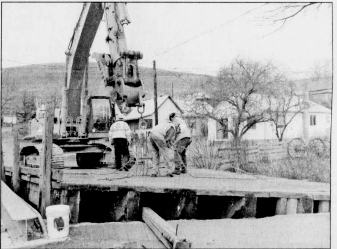
City workers, with the help of Knife River Construction, remove the old bridge on Quaid Street in Heppner. The bridge was replaced with a new structure. -Photo by David Sykes
