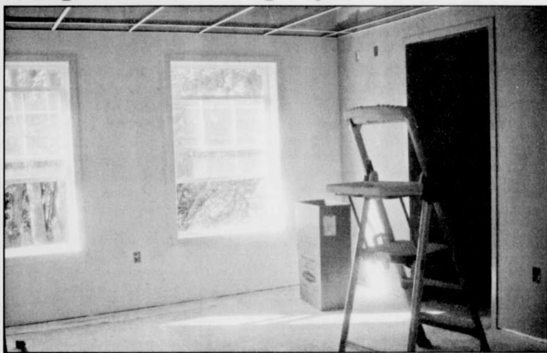
The remodeling project underway at Pioneer Memorial Hospital is "on schedule," according hospital CEO Victor Vander Does. The remodel, which includes three private rooms, two semi-private rooms, a tub room, and a solarium/dining room, should be finished around mid-November. The changes were made to accommodate a long term care facility. -Photo by Autumn Morgan
