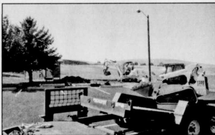
The Willow Creek Park District is putting in new bathrooms at the Willow Creek Lake. Concrete pre-fabricated bathroom will be put in on Thursday with a sidewalk around them. -Photo by David Sykes
