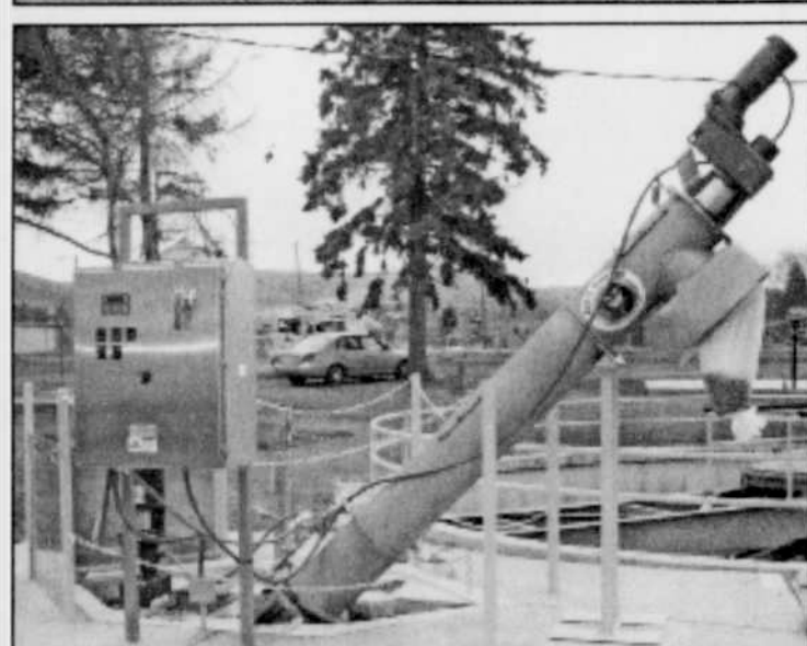
Top photo: The old propane generator. Middle Photo: The new generator. Bottom Photo: The Auger Monster that will break down solids. -Photos by Autumn Morgan
