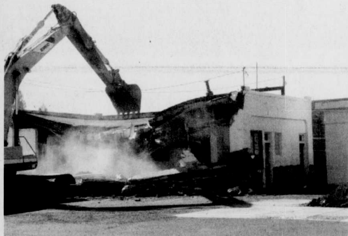
The old mini-mart across from Bank of Eastern Oregon was in the process of being demolished on Tuesday, April 25. In its place, Wheatland Insurance will be building an office building, said Jim Swanson, owner/partner of Wheatland Insurance.
