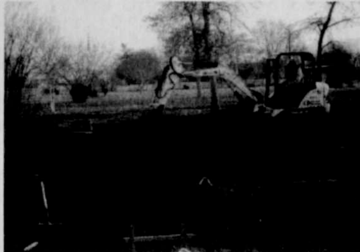
Ione Maintenance Supervisor Steve Dumler works at preparing the area for new public restrooms in Ione.
