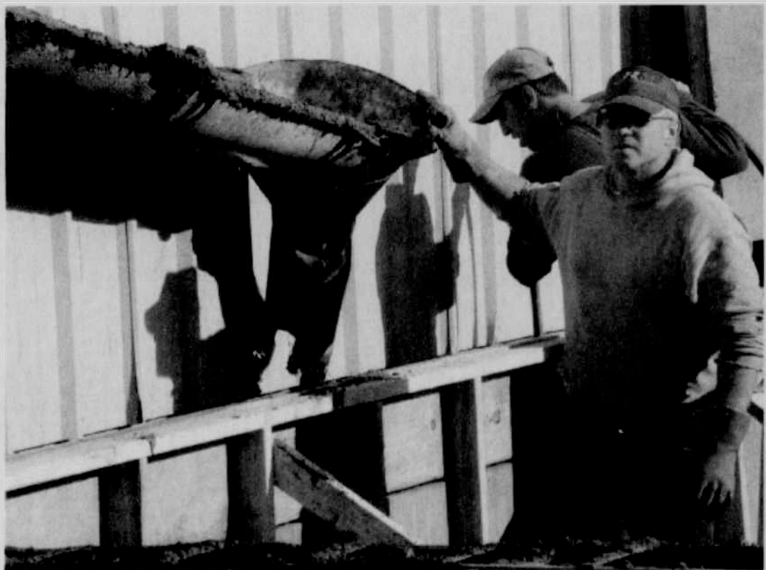
Jerry Gentry (front) of Gentry Home Improvements and employee Joey Hoffman work on the CSEPP building going up in Heppner.
