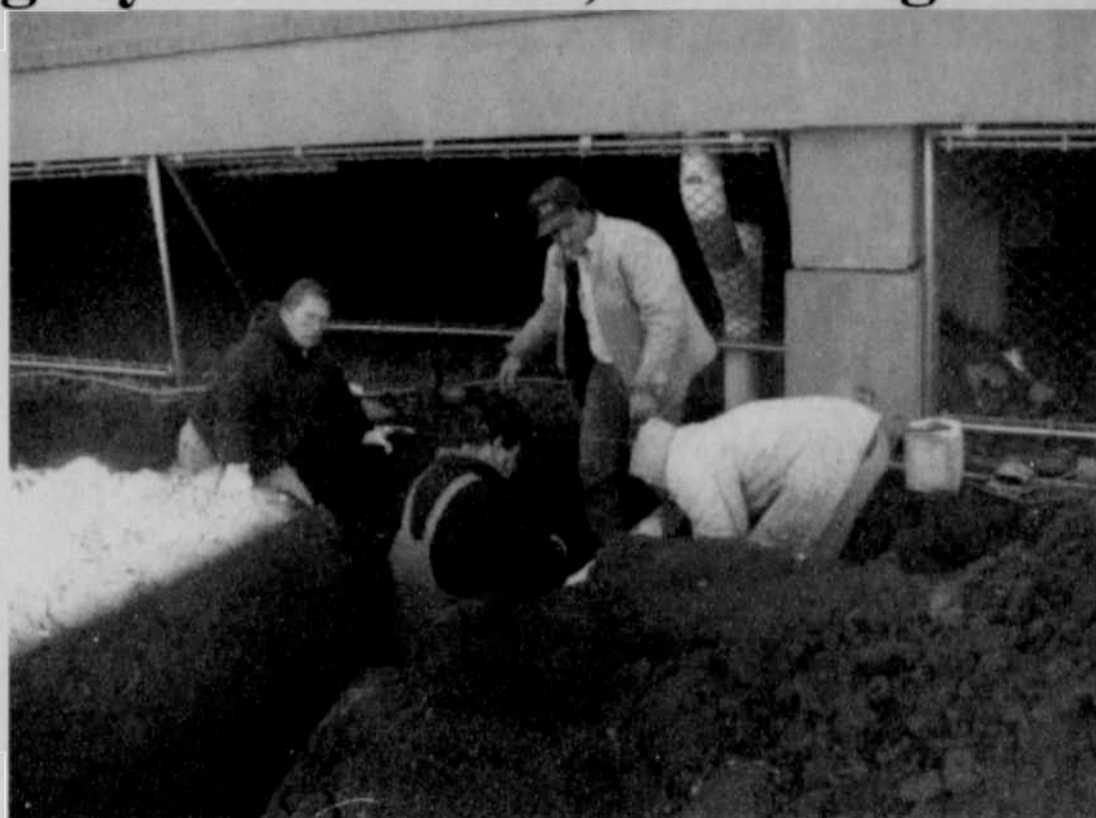
(L-R): Arlynda Gates, Ken Klinger, Keith Morter and Conrad Tworek hook up drain pipes from under the school building.
