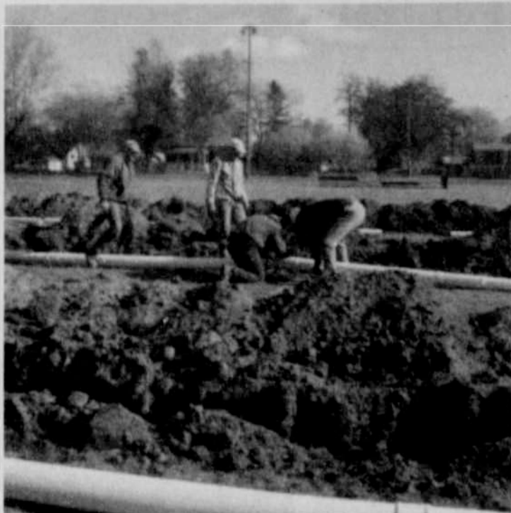
(L-R): Kevin Haguewood, Dustin Haguewood, Joe Rietmann and Jim Swanson connect drain pipes together.
