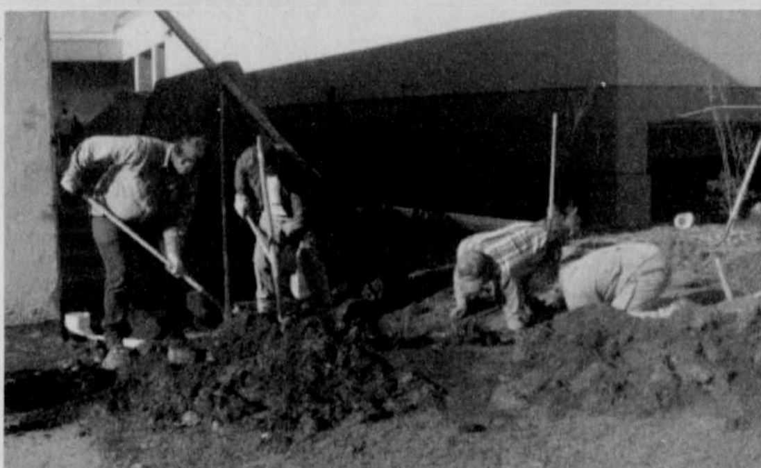
(L-R): Joe Orem, Del LaRue, Eric Orem and Gregg Rietmann work at laying the drain pipes.
