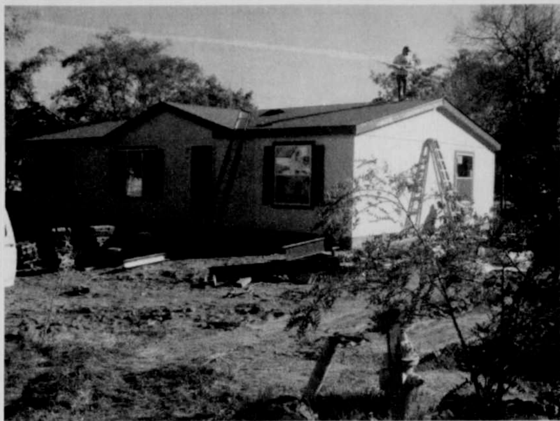
A new manufactured home is being installed on a Water Street lot left vacant by fire last year. Workers are currently working on completing the set up process of the house.
