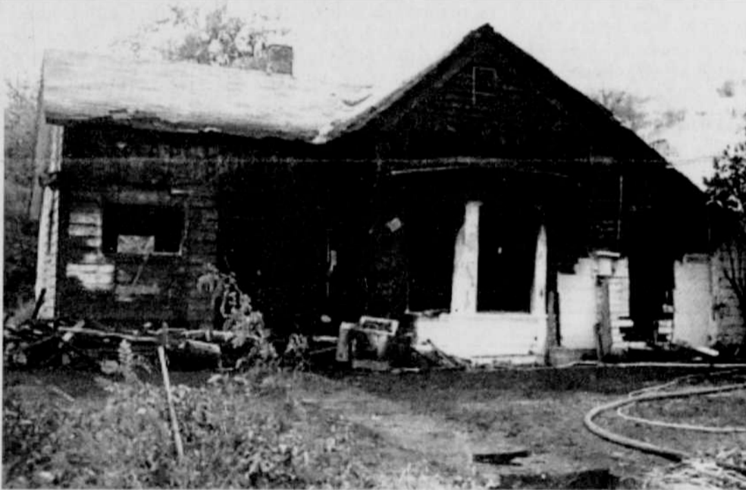
The remains of the home of Dale and Diane Munkers on Water Street in Heppner.
