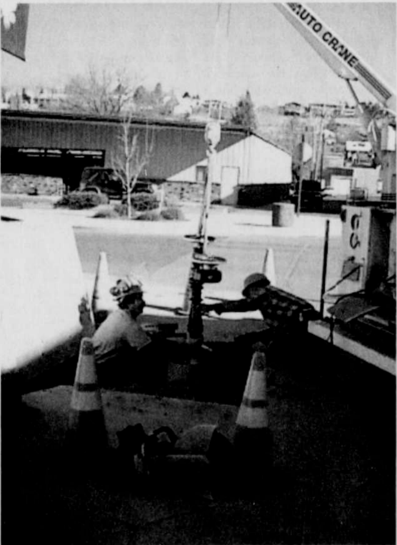
Craig Canham (left) and Roger Ehrmantraut work on installing a new water fountain at the corner of Main and Willow in Heppner. The fountain was donated to the city by the St. Patrick's Committee in memory of the Irish settlers in Morrow County. The fountain will be dedicated St. Pat's weekend, Friday, March 14.
