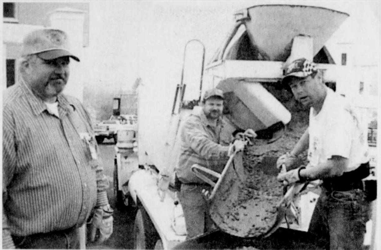
(L-R): Rusty Estes, PMH maintenance supervisor, Ryan Miller, and Mike Doherty, PMH maintenance
