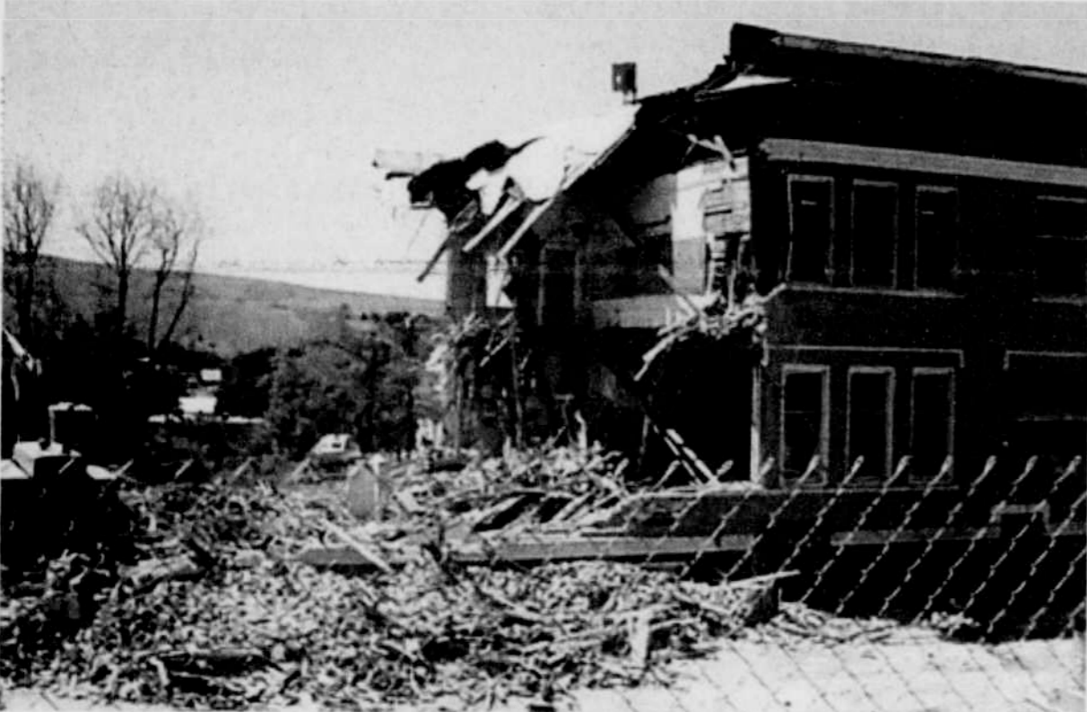
The old Heppner High School building is being torn down by McCormick construction of Pendleton.
