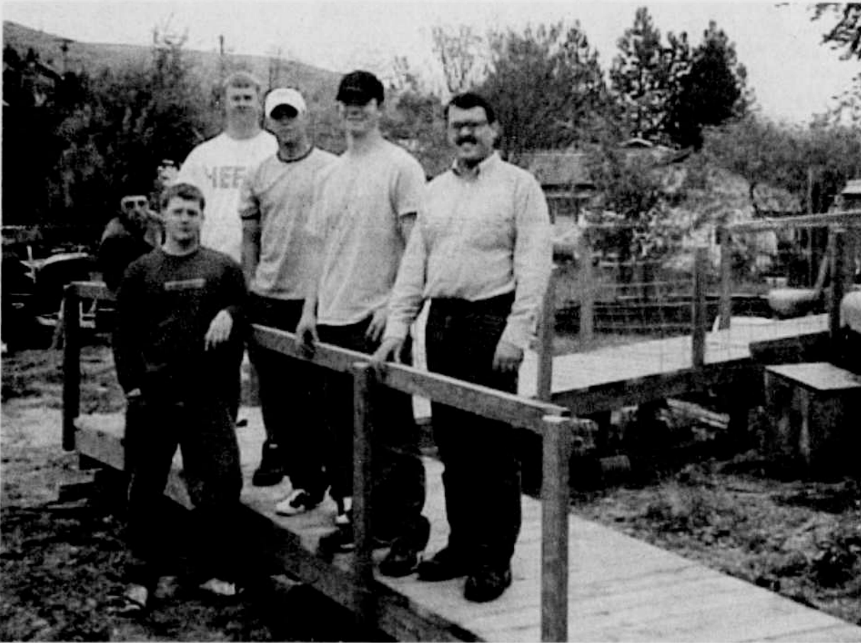
Dave Fowler's Construction Technology class built the wheelchair ramp as a class "real type" project.
