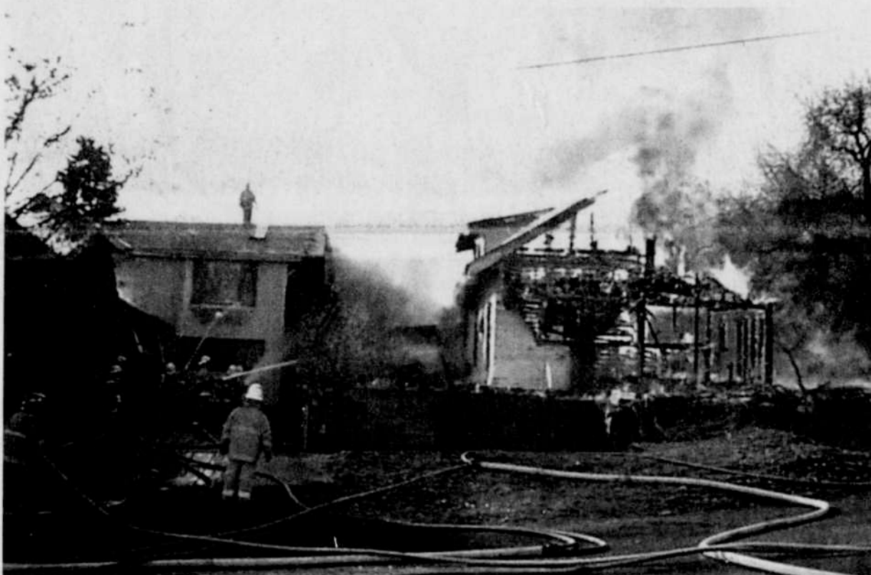
Practice burn The Heppner fire department, along with other area fire departments, conducted a practice burn Saturday. The house was located on West Willow Street in Heppner and the burn went off without any major problems.
