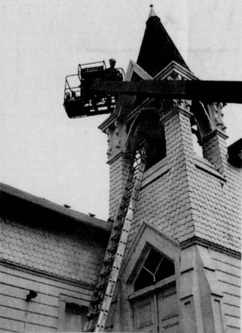
Rick Drake does his own version of a high-wire act as he repairs the steeple roof at the Heppner United Methodist Church this week.
