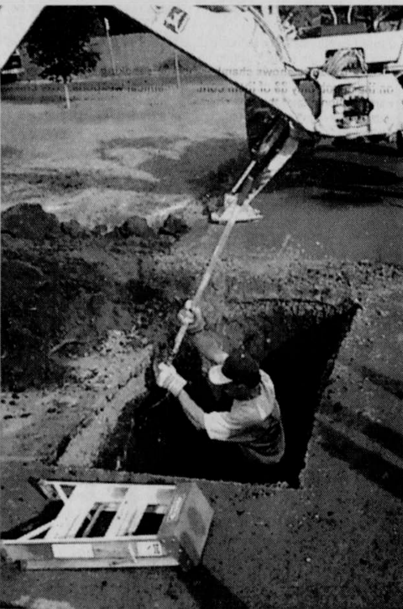
Heppner city crewmember Randy Sample prepares for placement of new valve on a city water main on Riverside street last Thursday. The new valve (along with a second valve) will enable city crews to shut down water to just part of the city. Previously for work to be done or in the event of an emergency, water to the entire city would have to be shut off, says city Manager Jerry Breazeale.
