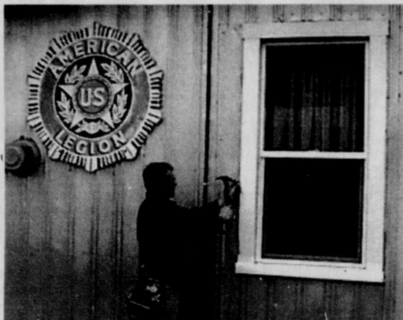
Blu Blakely, of Blu Blakeley Construction, installs a window at the lone American Legion Hall. The hall is undergoing renovation with funds received from a Fred Meyer grant.
