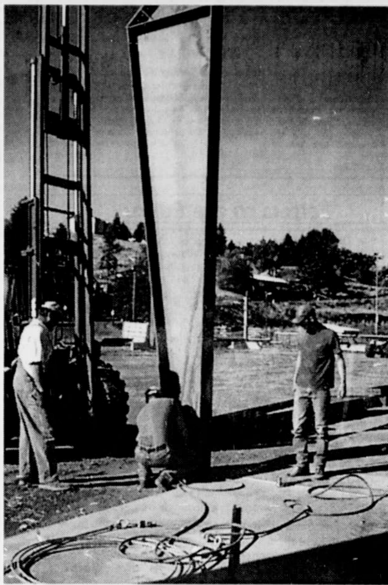
Volunteers began putting up the framework on the Wilkinson arena at the Morrow County Fairgrounds in Heppner last weekend. A crew is expected to put up the siding in mid October. Those volunteering Sept. 12 included Greg Close, Burrell Cooley, Jim Lunders and Jimmy Lunders, all of Irrigon, Ron Baker, Boardman and Tim Griffin, Prime Equipment and N.W. Metal Fabricators, both Hermiston, and Baker Hay Co., Boardman, donated equipment.
