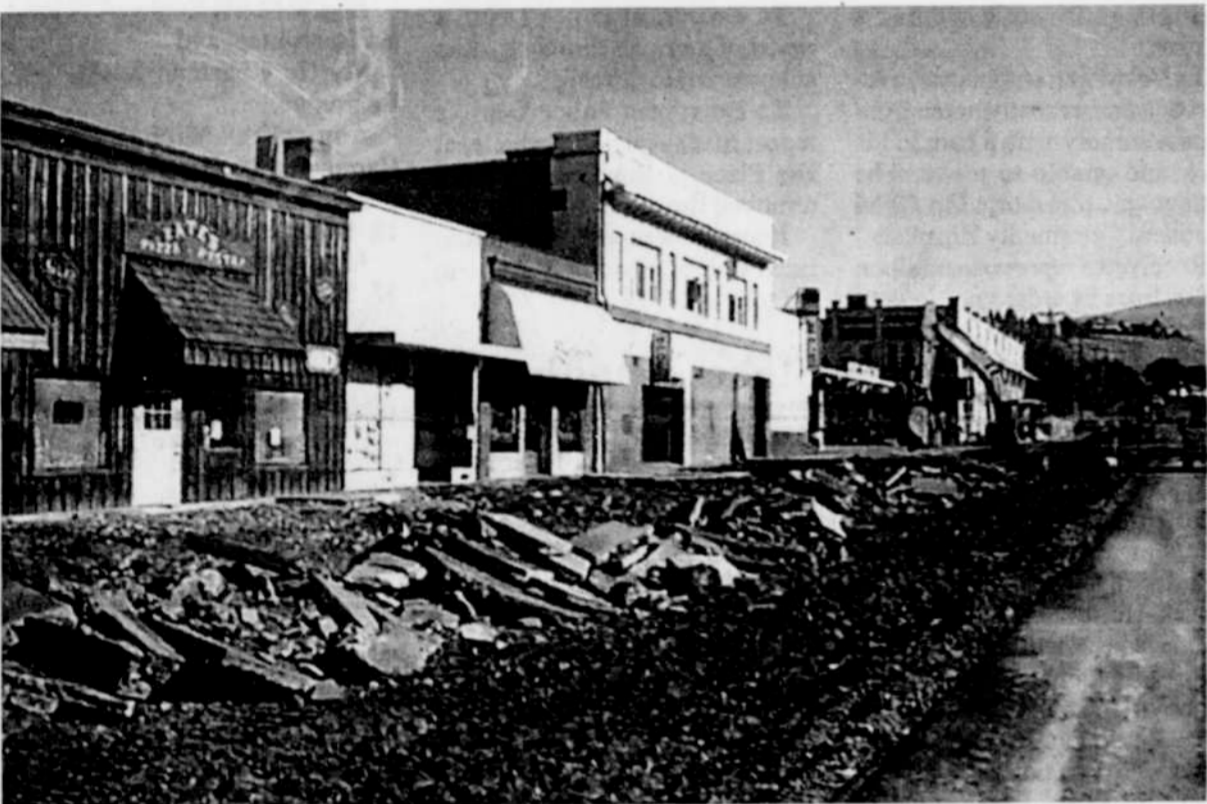
Following the Morrow County Fair and Oregon Trail Pro Rodeo Main Street Parade down Main Street Saturday, construction got underway this week on the east side of Main Street. Crossing the street Tuesday often proved difficult for pedestrians and motorists alike.
