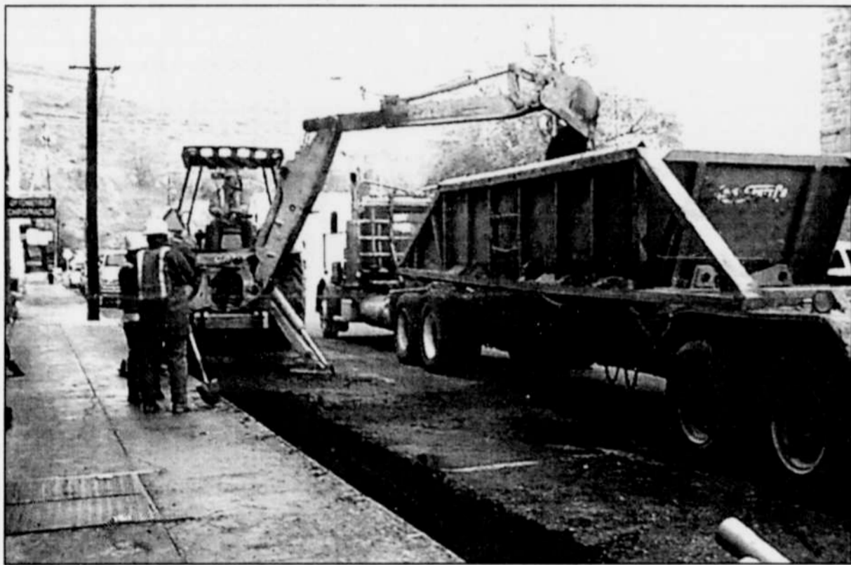
PTI workers continue work this week putting in underground cable in Heppner in preparation for the Main Street renovation project. PTI plans to begin work next on the street by the BP Station.
