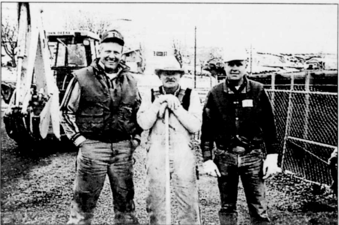
Morrow County Fair Board members (L-R) Alan Holmes, Joe Yocum and Sam Bellamy pause from work on the fairgrounds new water line.
