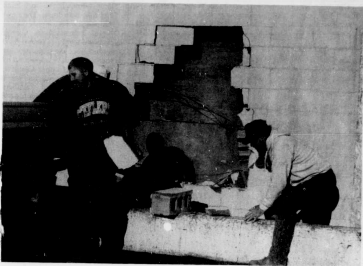
Jeff Orr (left) and Ken Eckman, of Eckman Construction, prepare to close up wall damaged by logging truck
