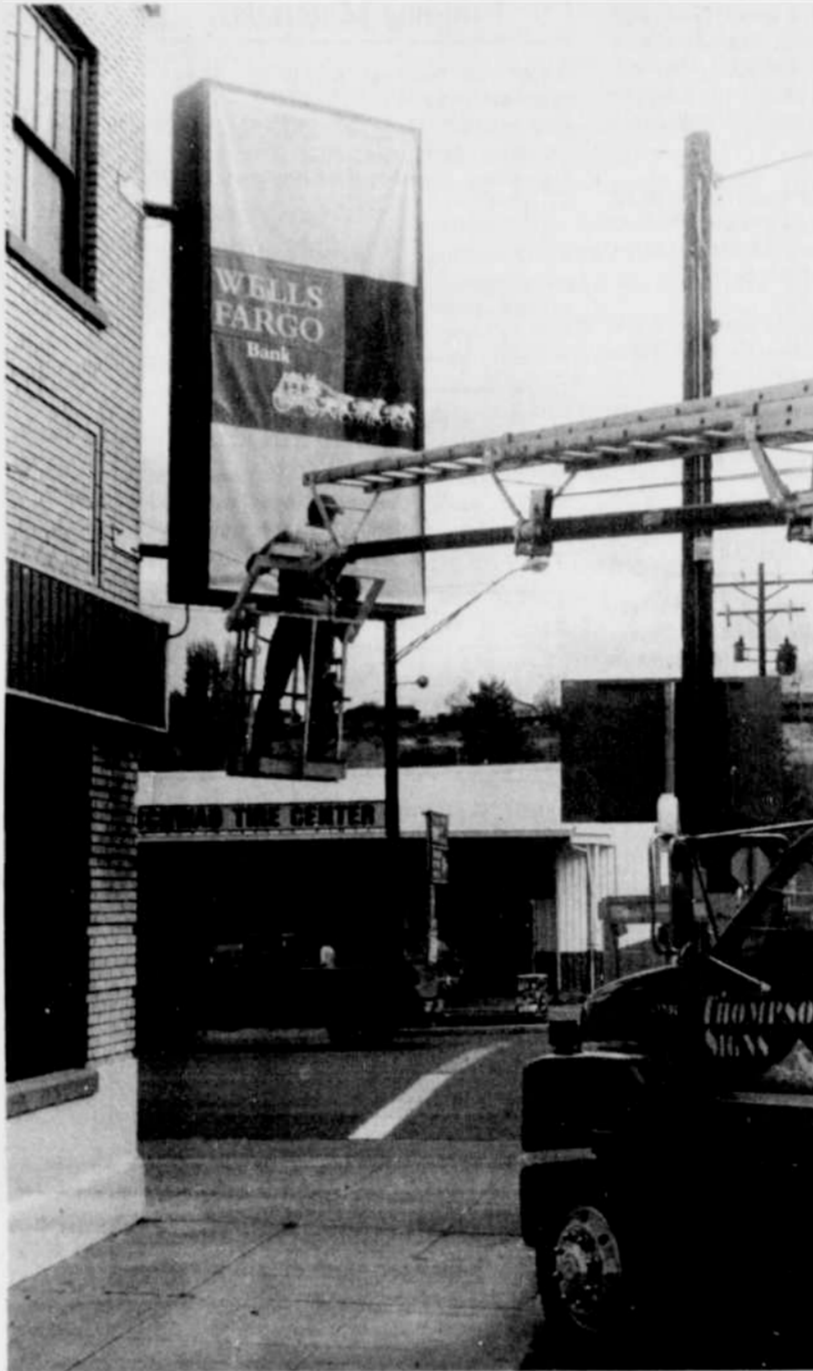
The sign at Wells Fargo Bank in Heppner, formerly First Interstate, got a facelift Tuesday, Nov. 5.
