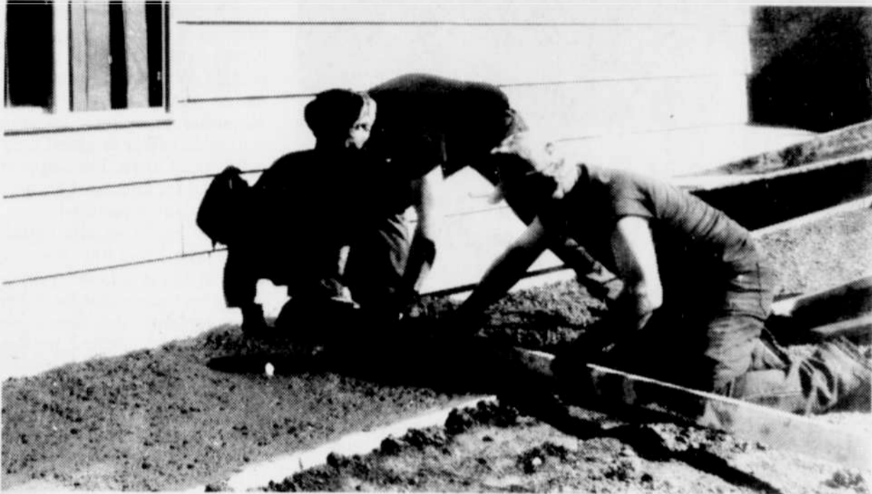
Gary Watkins and Simon Winters prepare cement walkway and ramp for the Doherty home.
